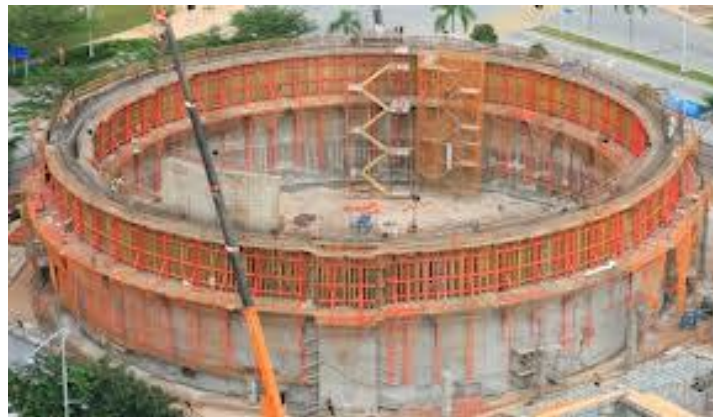
Fig .1.3: Clear Water Reservoir
